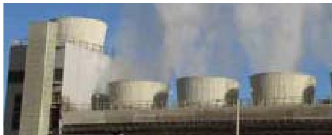
Figure 29. San Juan generating station
